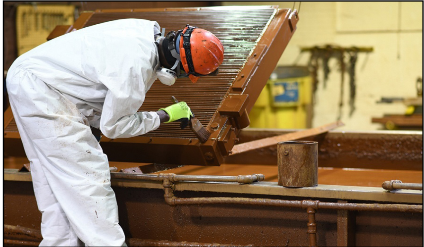
Traditional corrosion protection can disrupt your business or home comfort. Units are disassembled and transported to a facility for coating, leading to days or even weeks of downtime.
